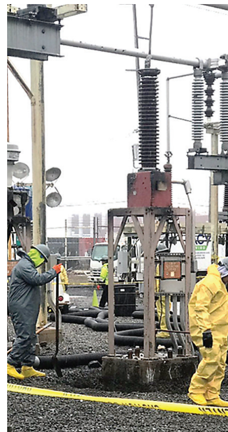
Failed CCVT with C1 Stack missing
